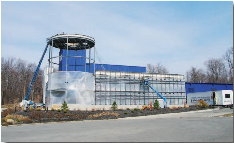
Offices under construction, the third phase of a $4.2 million project located in Lexington Industrial Park in Lexington, Ohio.
